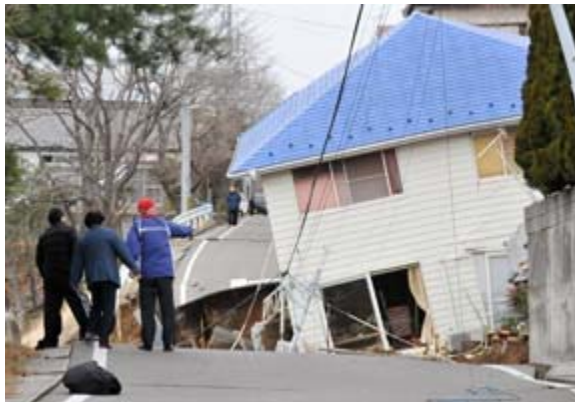
Residents check the damaged done on a road and house in Sukagawa city, Fukushima prefecture in northern Japan on March 2011, FUKUSHIMA MINPO/AFP/Getty Images
